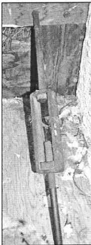
Left: Typical turnbuckle installed to link wall plates (top) with beams below (one of four).
